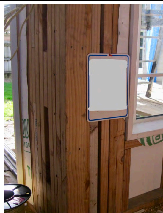
High concentration of corner framing leaves this external corner almost completely uninsulated
