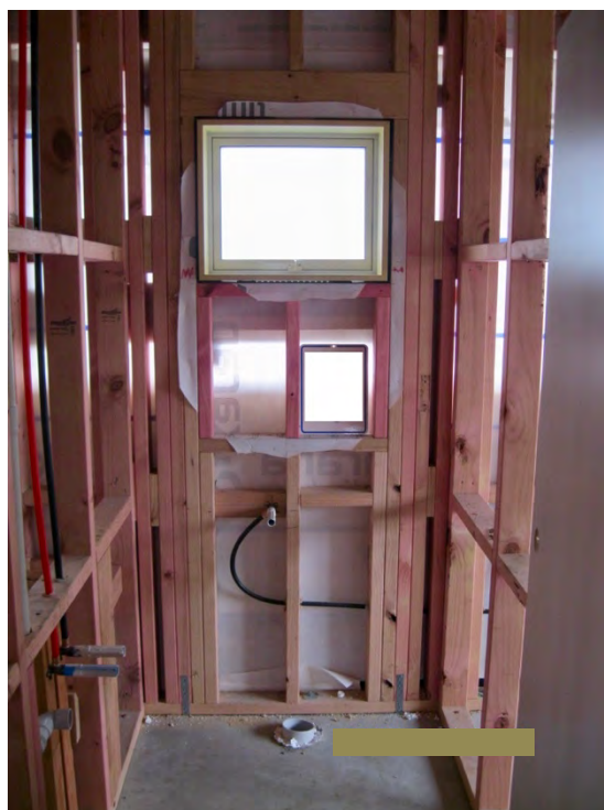
Two internal wall junctions in a small toilet wall next to an opening. This results in a high percentage of framing in this wall – in an area that may be prone to condensation
