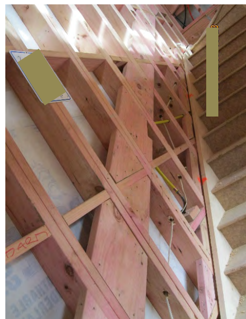
Photograph taken looking up the stairs and showing a large expanse of added blocking to take a handrail
