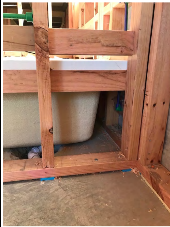
An uninsulated wall behind a bath – in this case the timing of the trades works against this being insulated properly
