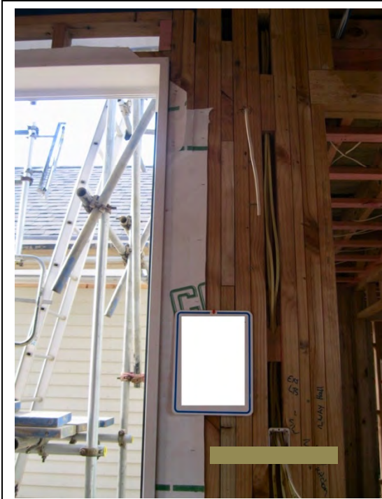
An example of a five-stud corner next to multiple trim studs to account for the window opening
