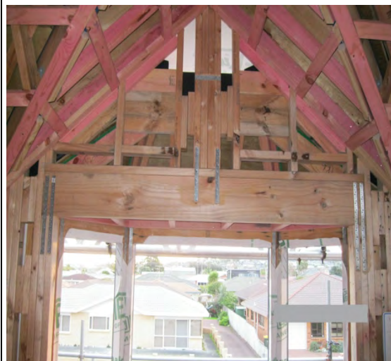
High concentration of framing and a combination of difficult shapes making insulation difficult
