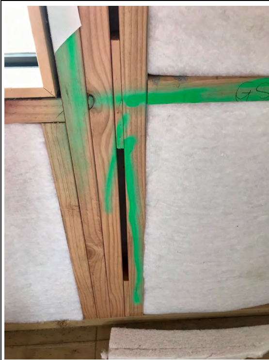
An example of timber fillet packing in the framing which leaves an uninsulated gap in the thermal envelope
