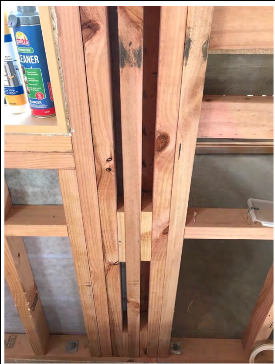
An example of packing in the framing which mitigates against getting insulation into these small and inaccessible spaces. Spray in expanding foam may be the only solution in these areas
