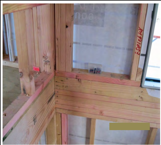
A built up section of midfloor indicating the extent of the uninsulated solid timber thermal bridge (approximately 410mm) created between the two levels
