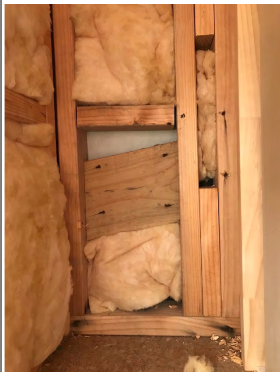
140mm blocking on edge to support flashing for the apron roof – noting that the 45mm face remains uninsulated as well as the awkward gap left behind in the space above it
