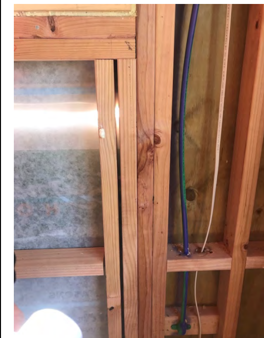
This gap between these two studs will be hard to fill with insulation and will be a significant source of heat loss in this section of the wall
