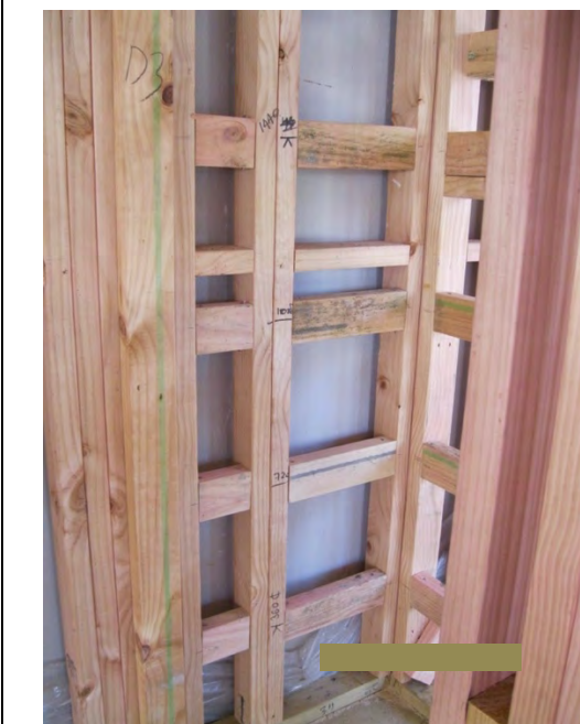
The effect of added blocking to support shelving in a cupboard space – note also the uninsulated internal to external wall junctions
