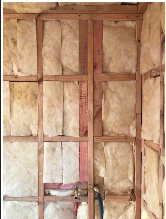
90mm blocking on edge to take plumbing pipe fixtures – the 45mm space behind this edge fitted timber remains uninsulated
