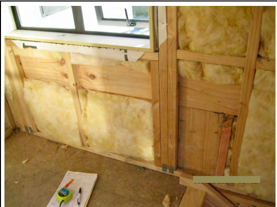
A large area of blocking added across several wall panels to take an apron roof flashing
