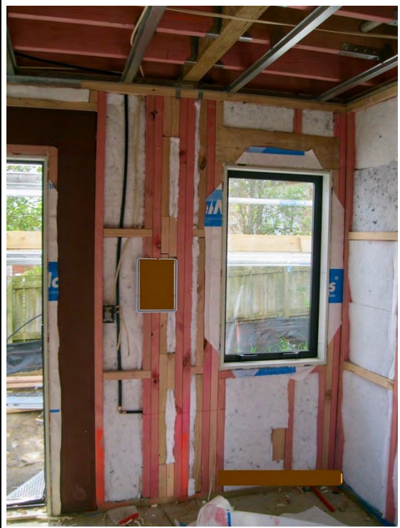
Large steel portal (uninsulated) around door and adjacent to a wall with a high percentage of framing
