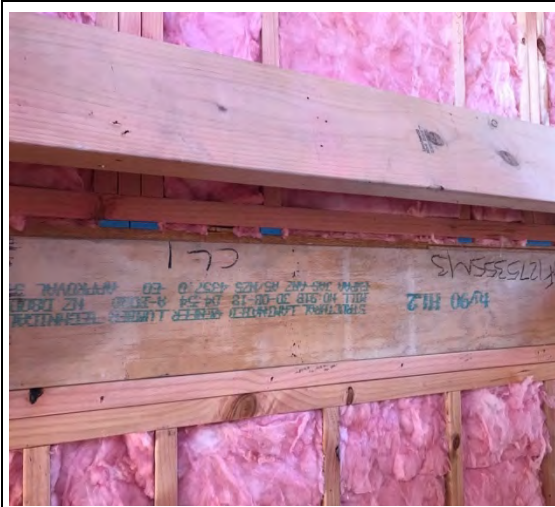
A midfloor section (photographed from within the stairwell) indicating the large uninsulated 'ribbon' right around the house between the two floors
