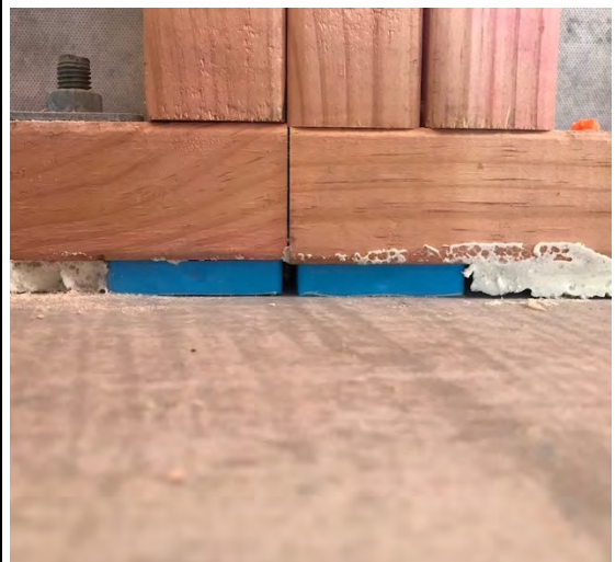
The plastic packer under the bottom plate – in this instance with gaps and less than adequate expanding foam under the full width of the bottom plate
