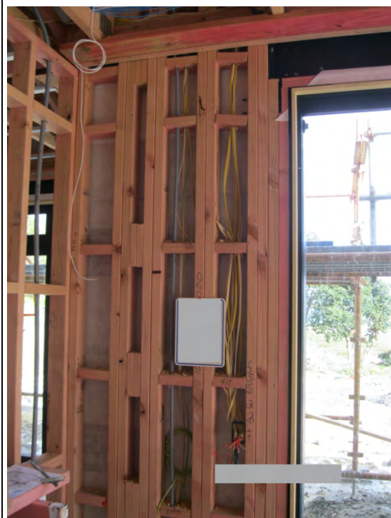
A high percentage of framing with close noggling, blocking and multiple studs next to a large window
