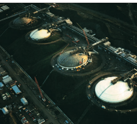
Liquefied natural gas separation plant at Mossmorran, Scotland. Insulation for the bases of 4 LNG and LPG tanks, pipework and various equipment (operating temperature: -160°C to +175°C).
